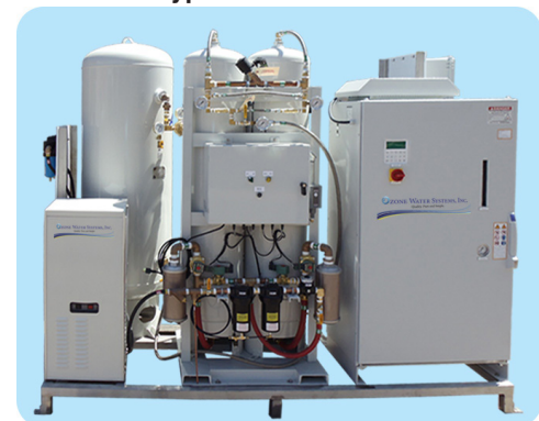
Typical Ozone Skid
